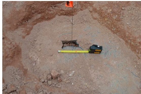
Figure 6. Rock Puncture damage.
